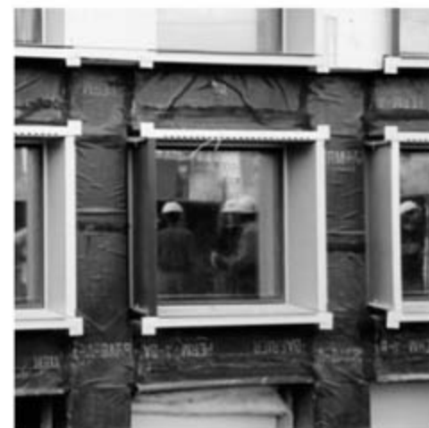
Fig. 2. Detail of an unfinished exterior wall assembly showing a waterproof membrane of self-adhering ethylene propylene diene monomer rubber (EPDM) on a structure of precast concrete inset with aluminum window frames. [Photo by J. E. Fernández]
